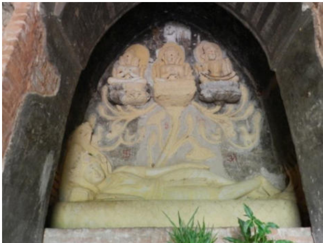
Plate 3.6: Brick and stucco relief of a reclining Vishnu after renovation at the principal niche, Nat-hlaung Kyaung temple, Pagan.
