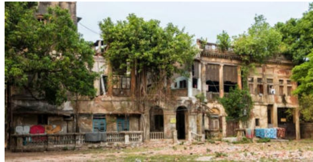
Plate 17.19: Recent photograph of the shabby and deplorably ruined condition of the House of the Nawab at 85 Park Street.
