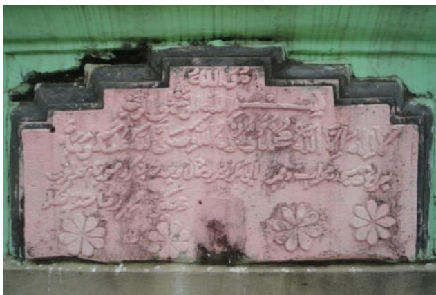
Plate 11.30: Farsi Inscription of the original mosque embedded on the parapet of the structure.
