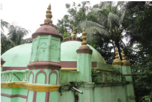
Plate 11.34: Blind kiosks of corner towers engaged turrets. The corner tower displaying merlon designs, moulding semicircular cusped arch design framed within rectangular panel. The finial exhibiting the lotus and kalasa motif but abstract in design.
